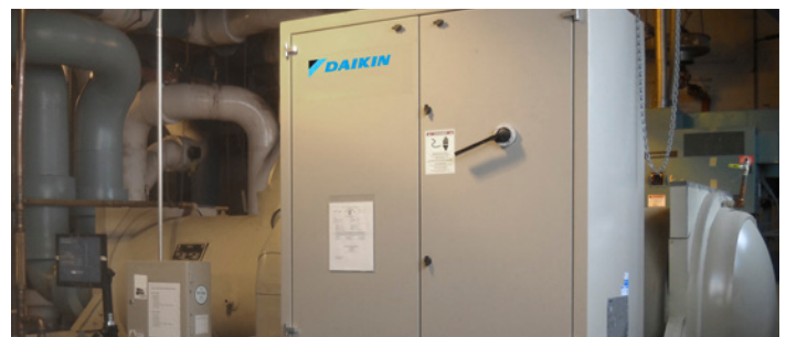
The Magnitude chiller installed at the Skyline Madison Campus is the latest of the many Magnitude chillers that HCA has installed in its healthcare facilities around the country.
