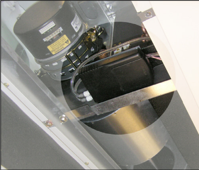
Figure 97: CO 2 Sensor For Demand Control Ventilation
